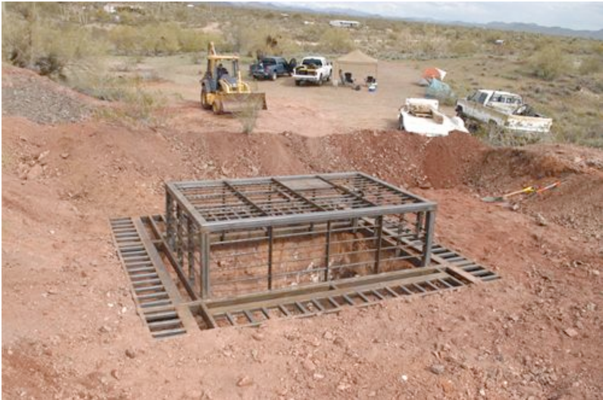
Installed Cupola Bat Gate
