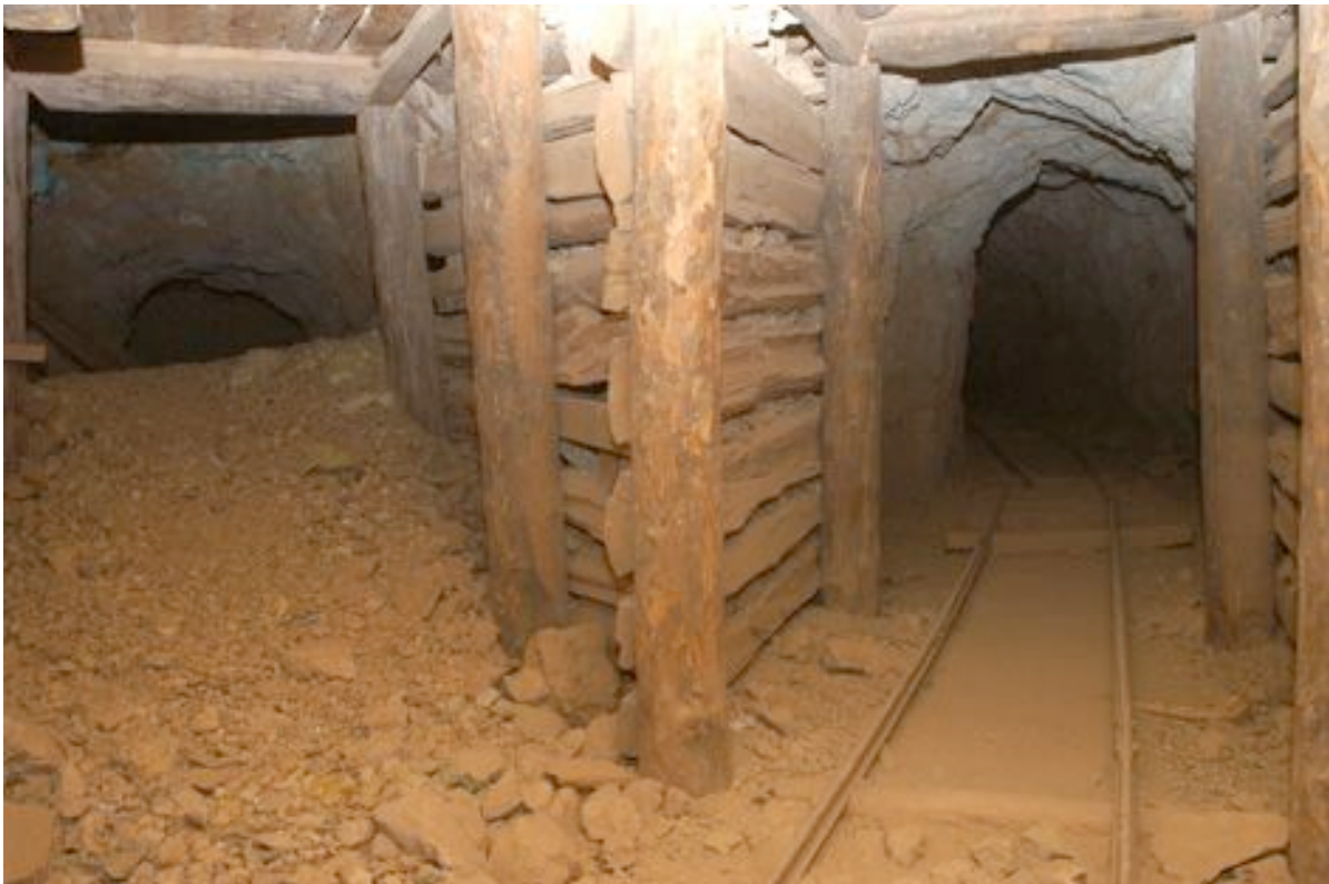
Collapsing Tunnel in Grandview Mine
